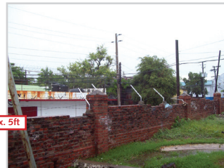
Photo 6: Low perimeter wall at the Elletson Road Station on September 30, 2013.
