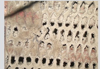
Photo 12: Blocked ventilation ducts at the Savanna-la-mar Station.
