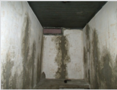
Photo 7: Blocked out ventilation in cell at Stewart Town Station.
