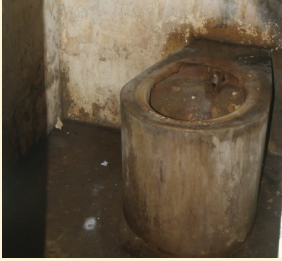
Photo 6: Non-functional toilet at the Savanna-la-mar Station lock-up.
