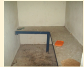
Photo 12: Cell at Glengoffe Station without bedding on bunk.
