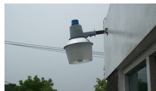
Photo 1: One of four perimeter lights out of service at the Fletchers Land Station as seen on August 13, 2013.
