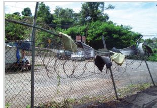
Photo 1: Defective perimeter fencing at the Red Hills Station as presented on November 5, 2013.
