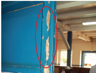
Photo 9: Rotting walls in the Mocho Station as seen on March 19, 2014.
