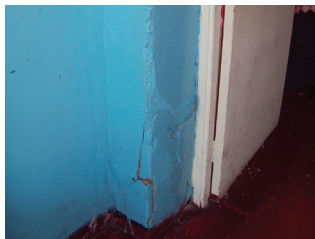
Photo 5 & 6: Cracks in the wall at the station.
