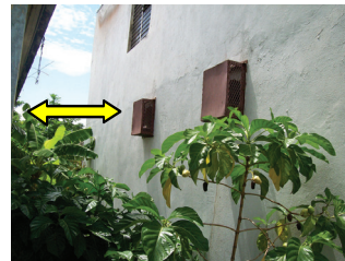
Photo 7: No perimeter fence between abandoned house and lock-up at the Mountain View Station as seen on September 27, 2012.
