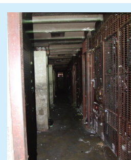
Photo 5: Hallway of lock-up at Spanish Town Station with dim lighting.
