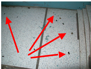
Photo 1: Rat droppings on the floor in the officers' barrack rooms as seen on August 20, 2013.
