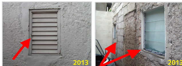
Photos 3 & 4: Windows still located in perimeter wall of neighbouring property of Allman Town Station in 2013.
