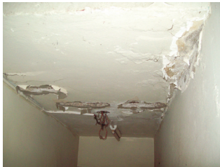
Photo 1: Exposed electrical wiring in unrepaired ceiling.
