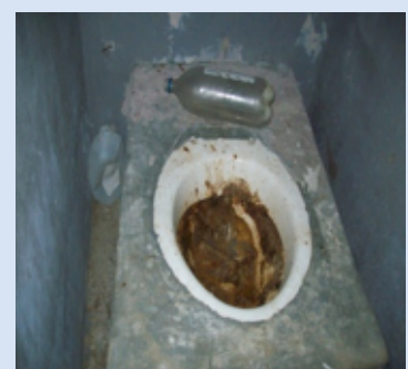
Photo 6: Clogged toilet in lock-up at the Frome Station.
