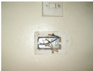
Photo 4: Uncovered electrical socket.
