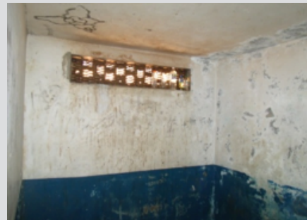
Photo 8: View of ventilation area with objects blocking it in cell at Barrett Street Station.
