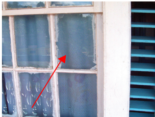
Photo 10: Broken pane in the window at the Mocho Station on March 19, 2014.
