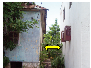
Photo 8: No perimeter fence between abandoned house and lock-up at the Mountain View Station September 24, 2013.
