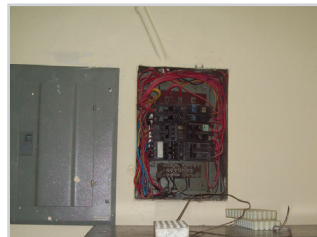
Photo 6: Exposed electrical wires at the Tivoli Gardens Post as seen on March 13, 2014.
