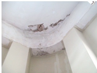
Photo 2: Cracks in ceiling showing exposed steel.
