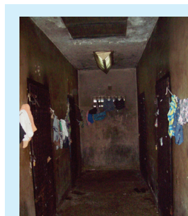
Photo 4: Hallway of lock-up at Montego Bay Station with dim light and articles of clothing strung over ventilation covers blocking natural light.
