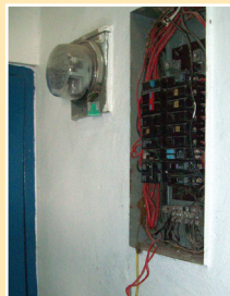
Photo 6: An open electrical panel at the Seaforth Station in 2012.
