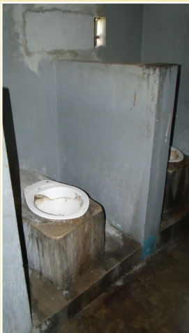
Photo 1: Non-functioning toilets at the Port Antonio lock-up as presented on May 15, 2014.
