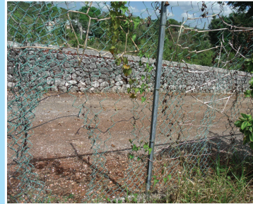
Photo 1: Poor perimeter fencing at the Cross Keys Station.
