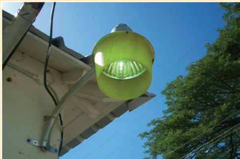
Photo 2: Security light on during the day at the Llandewey Station on November 25, 2014.
