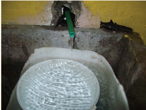
Photo 1: Makeshift pipe (hose) at the Seaforth Station as seen on November 27, 2014.
