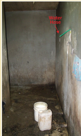
Photo 2: Converted shower area at the Port Antonio lock-up with buckets to catch water as presented May 15, 2014.
